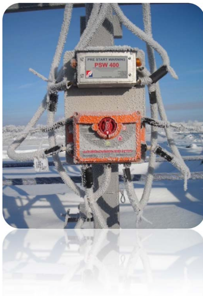
Conveyor Control Station - CCS
